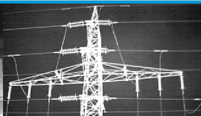
High voltage power lines
